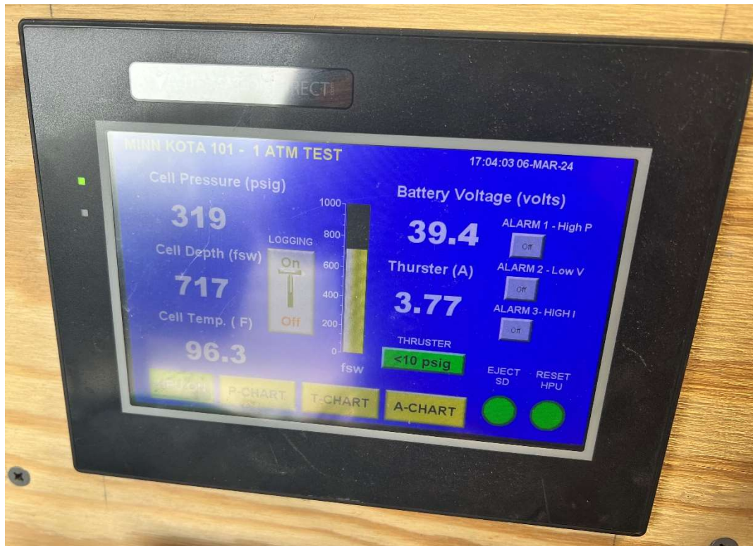
Figure 10 – HMI Home Screen - AutomationDirect C-More EA9-T7CL-R
